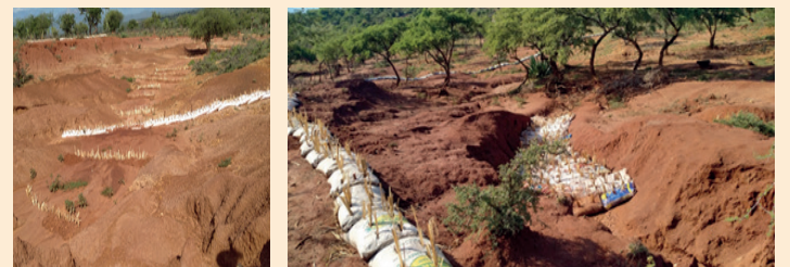
Gullies being rehabilitated at the Livestock Café sites in Chepareria Ward (Photo by M. Nyaga)
